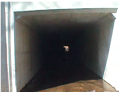
Figure 9. Culvert almost completely covering an unnamed tributary in the Middle Little Patuxent River subwatershed (site 069).
