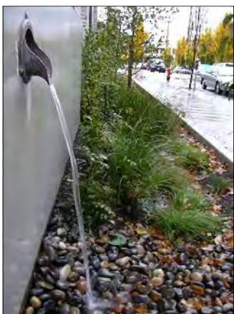
Rooftop Stormwater Treatment
