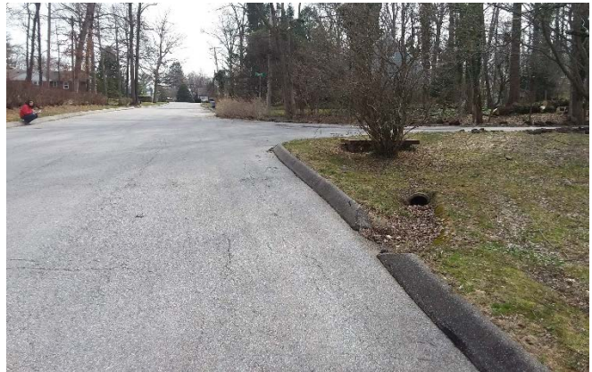
Figure 2: Opportunity to improve existing conveyance system along Underoak Drive.
