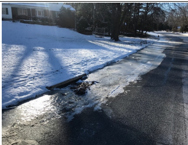
Figure 1: Ice buildup behind inlet at Michaels Way and Longview Dr.
