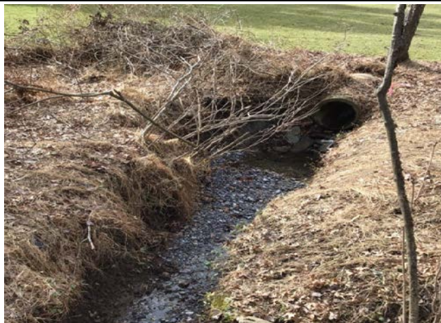
Figure 1: Unstable outfall and disjointed pipe section at outfall.
