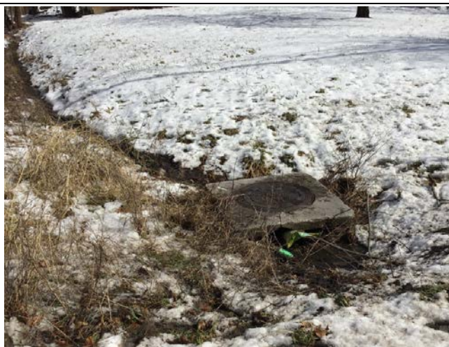
Figure 1: Stormdrain outfall channel with standing water leading to existing inlet.
