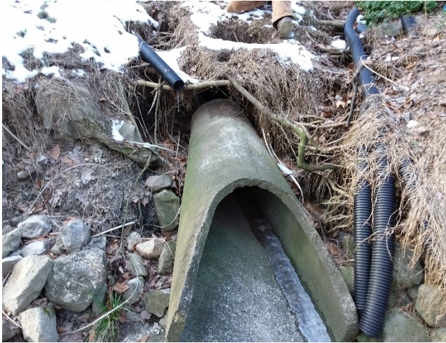
Figure 1: Outfall with detached end section requiring repair.
