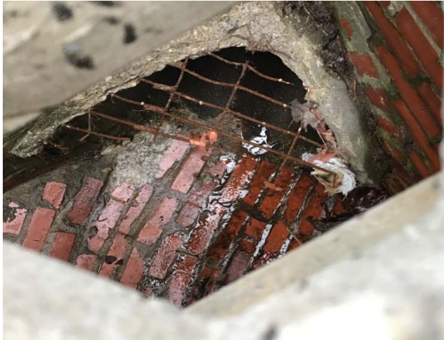
Figure 1: Exposed rebar in pipe.
