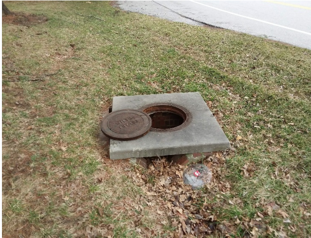
Figure 1: Typical inlet along Columbia Road.
