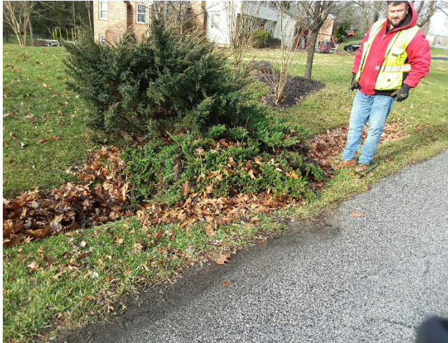
Figure 1: Inlet along Spring Meadow Drive with observed debris and vegetation.
