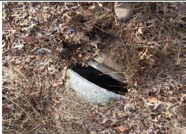
Figure 2: Disjointed pipe at outfall.
