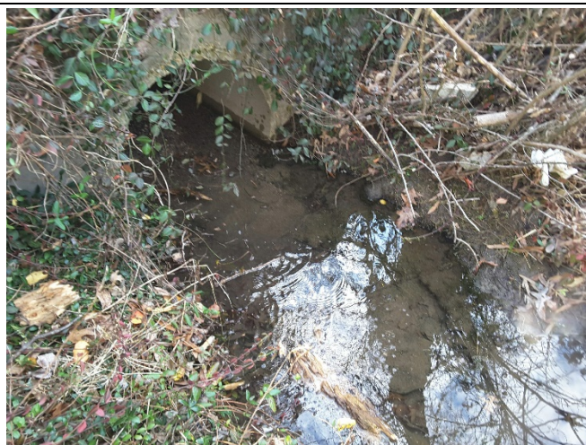
Figure 2: Typical pipe and outfall with observed debris.
