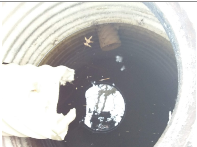
Figure 4: Pondered water within inlet along Chatham Road requiring further investigation.
