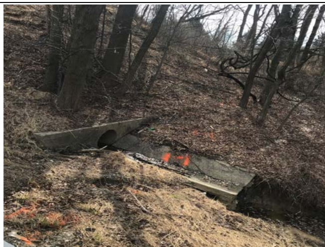
Figure 4: Severe erosion in the outfall channel downstream of outfall.
