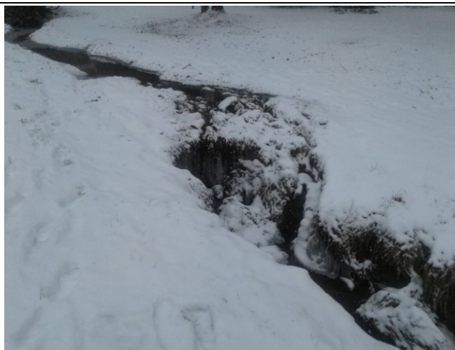
Figure 1: Significant erosion in outfall channel.
