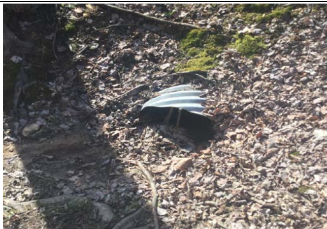
Figure 5: Outfall is deformed and partially buried.
