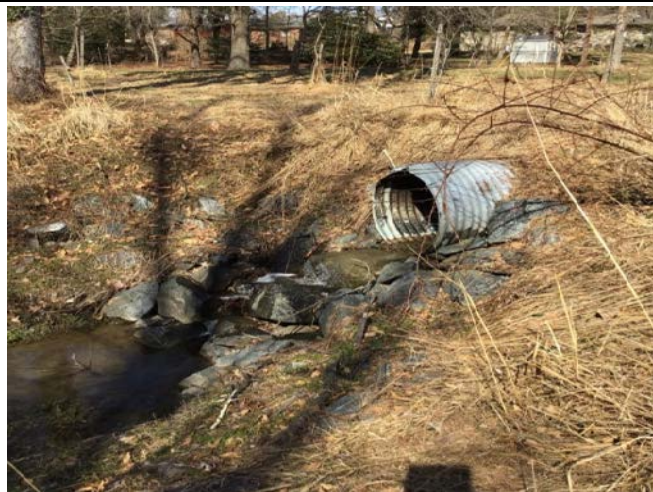
Figure 4: Outfall of storm drain network that is potentially inefficient.
