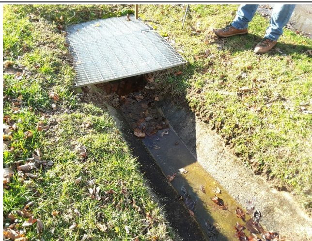
Figure 1: Typical inlet along Spring Meadow Drive.
