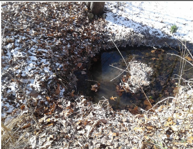
Figure 3: Outfall is submerged and buried.
