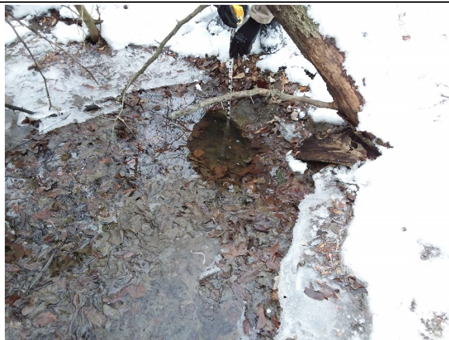
Figure 2: Typical submerged outfall requiring repair.
