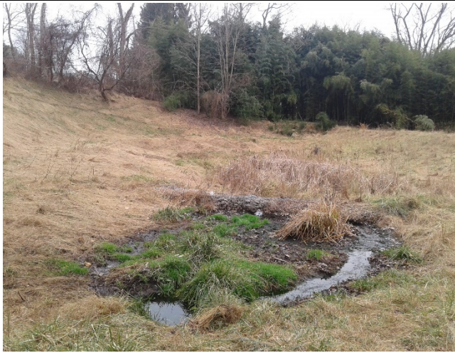
Figure 1: Pond forebay filled with sediment.
