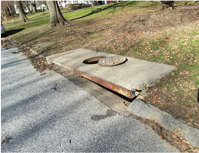
Figure 1: Damaged inlet along Dunloggin Road.
