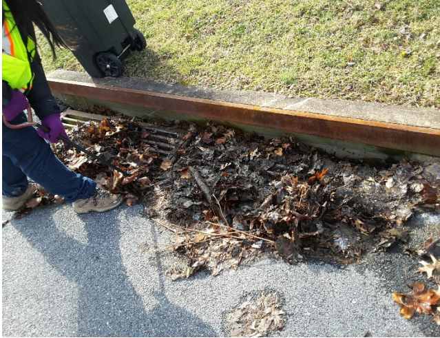
Figure 1: Typical inlet along Westwood Drive with observed debris.
