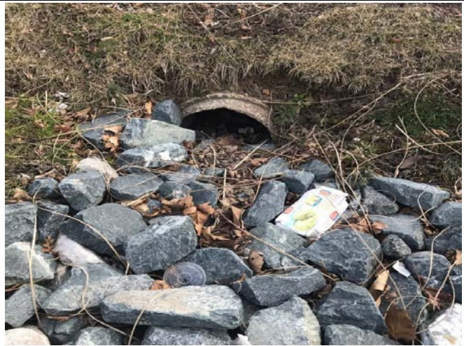
Figure 4: Outfall partially full with sediment.
