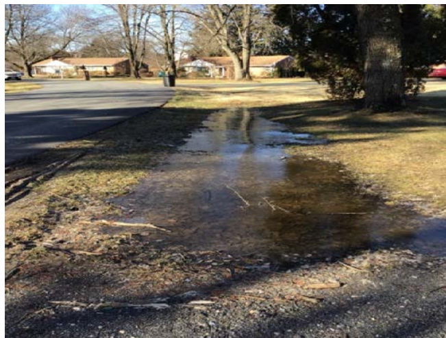
Figure 2: Standing water in roadside ditch along Millbrook Rd.
