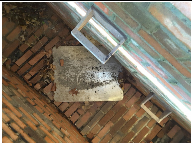
Figure 2: Typical inlet requiring repair along Nanmark Court.
