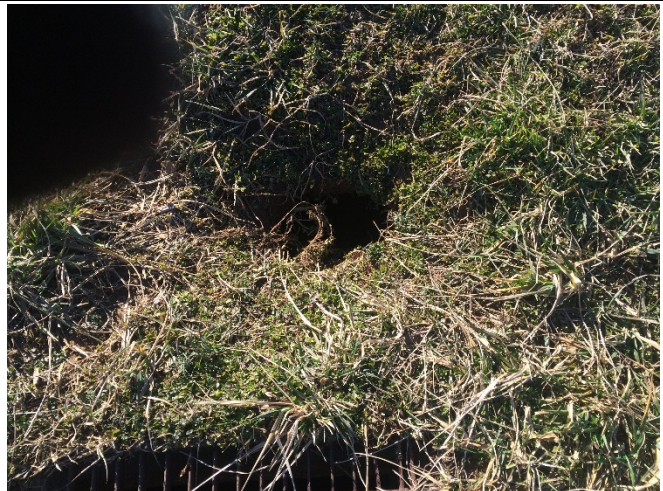
Figure 2: Sinkhole forming above pipe.
