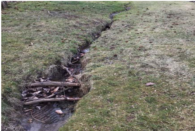
Figure 1: Outfall channel running behind back yard at 2802 Leaf Shade Drive is severely eroded.
