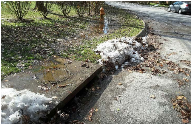
Figure 1: Opportunity to improve existing conveyance system along Underoak Drive.
