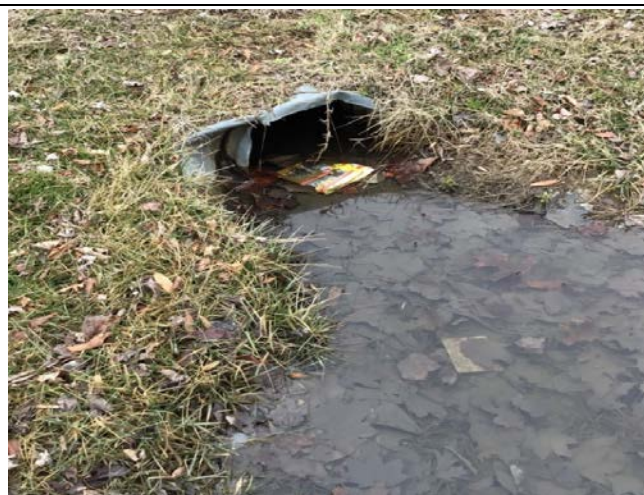
Figure 3: Outfall is deformed and deteriorating.
