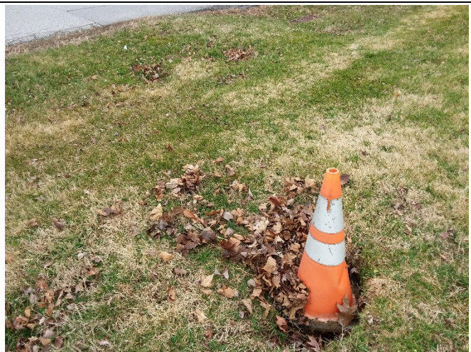
Figure 2: Sinkhole forming over pipe along Crestleigh Drive.
