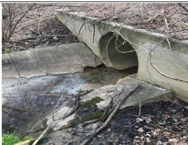
Figure 3: Erosion surrounding outfall channel of outfall.
