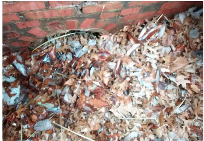
Figure 2: Inlet with observed debris.
