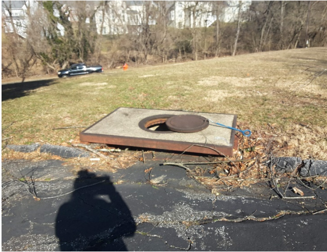
Figure 1: Inlet at Forest Hill Swim and Tennis Club requiring repair.
