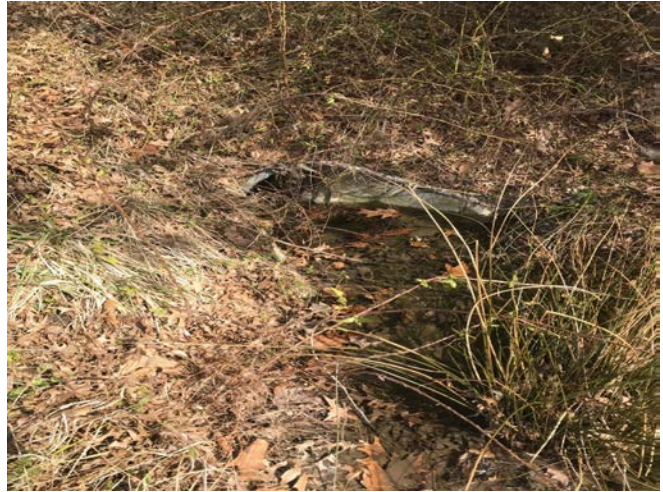
Figure 2: Outfall partially submerged.
