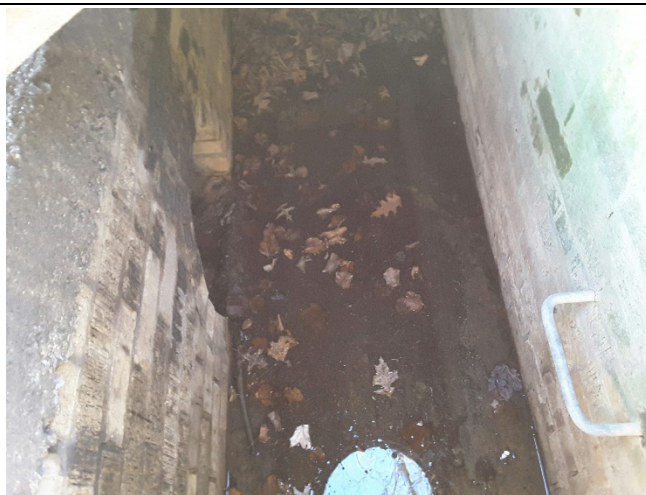
Figure 3: Typical inlet with observed debris along Plum Spring Lane.
