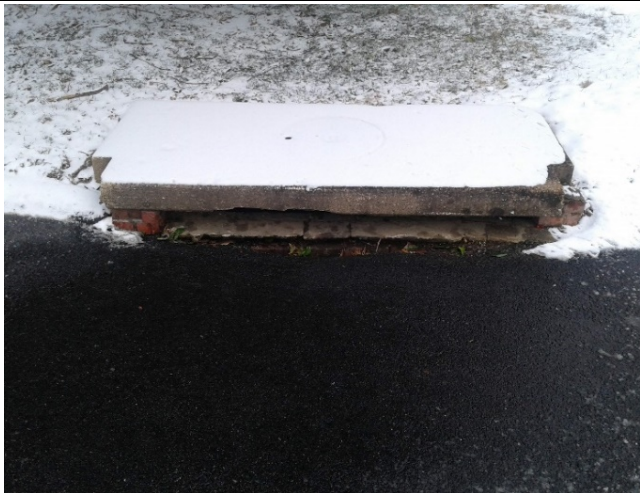
Figure 1: Damage along inlet opening.
