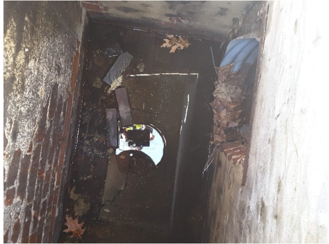
Figure 2: Inlet at Forest Hill Swim and Tennis Club requiring repair with observed debris.
