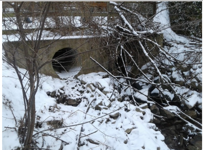
Figure 2: Branches partially blocking outfall.
