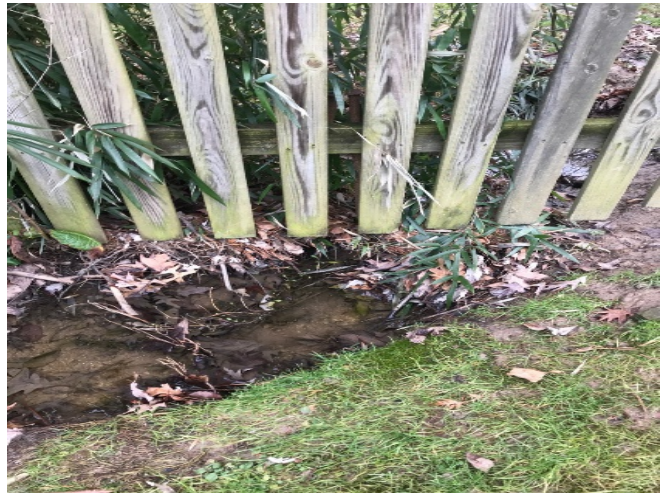
Figure 2: Standing water and sediment buildup under fence between 3134 Hearthstone Rd. and 9522 Joey Dr.
