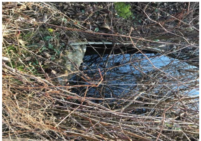
Figure 8: Outfall is partially submerged and overgrown with vegetation.
