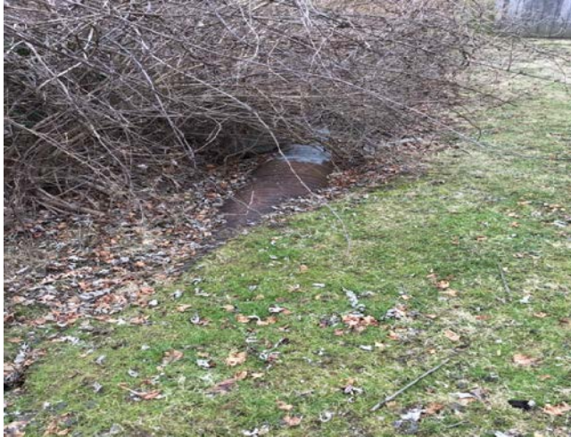
Figure 1: Storm drain top exposed.
