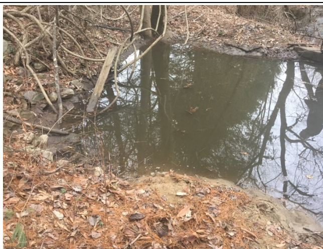
Figure 1: Outfall into pond unable to be located. Forebay is inundated with water.
