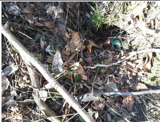
Figure 1: Outfall requiring repair.
