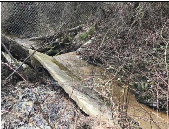
Figure 4: Erosion surrounding outfall channel, and damage to concrete channel of outfall.
