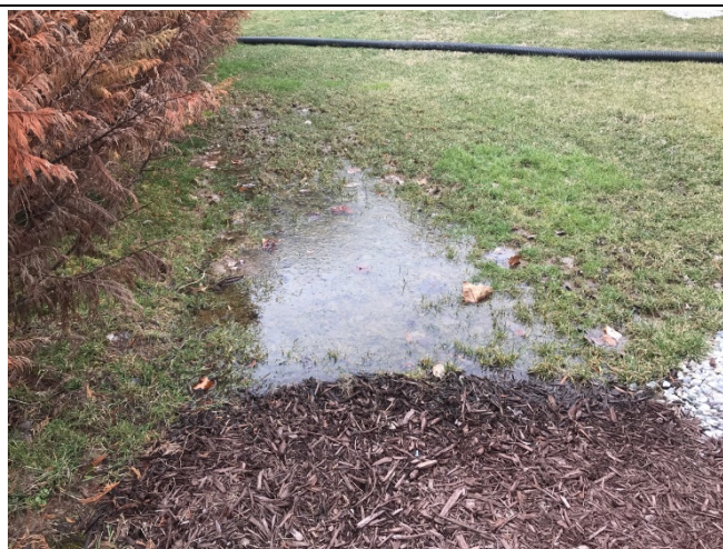
Figure 2: Localized ponding in area between houses.
