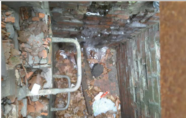
Figure 3: Typical inlet with debris along Baltimore National Pike (U.S. Route 40).
