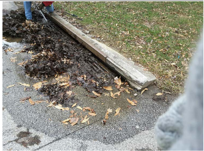
Figure 2: Typical inlet with observed debris along Dunloggin Road.
