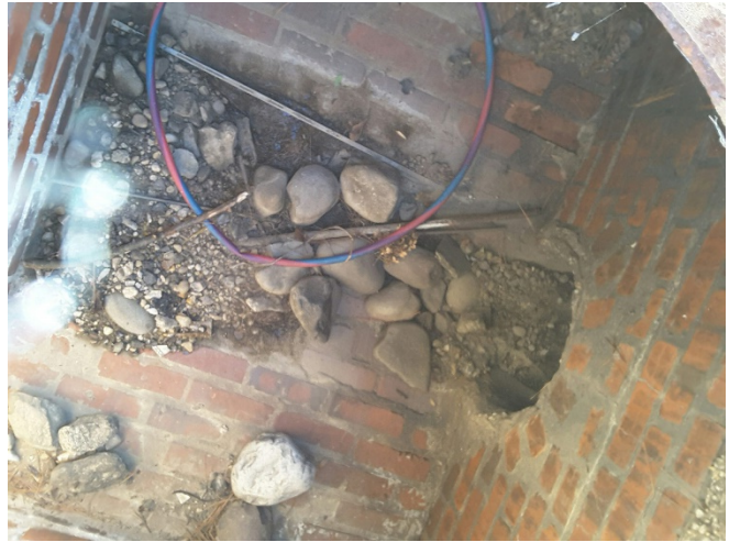
Figure 2: Typical inlet along Lowlen Court with observed debris.
