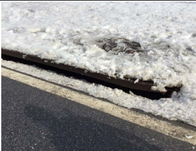
Figure 3: Damage on the front right side of inlet.
