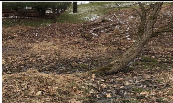
Figure 4: Buildup of sediment and debris at pond inflow.
