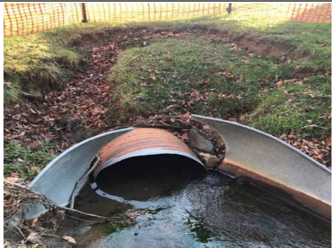
Figure 4: Disjointed end section at outfall and erosion is in the process of being repaired.
