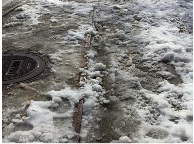
Figure 2: The back of inlet is raised, causing a safety hazard for pedestrians.
