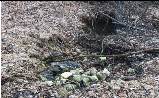
Figure 3: Significant erosion and debris in outfall channel.
