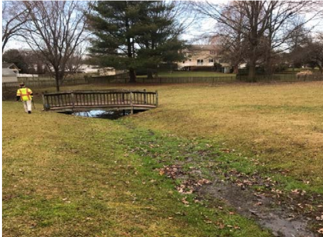
Figure 3: Eroded channel running behind house at 9522 Joey Dr.
