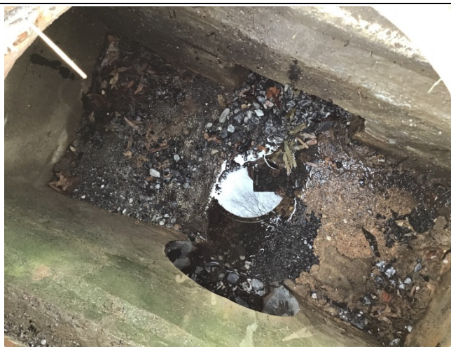
Figure 3: Gravel inside inlet.
