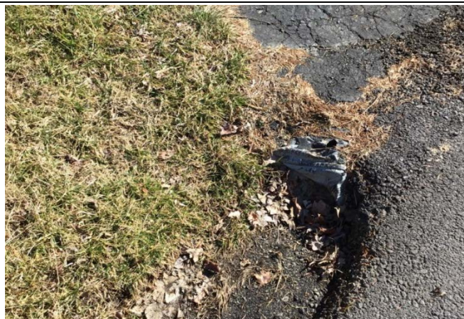
Figure 6: Outfall and associated pipe is damaged.
