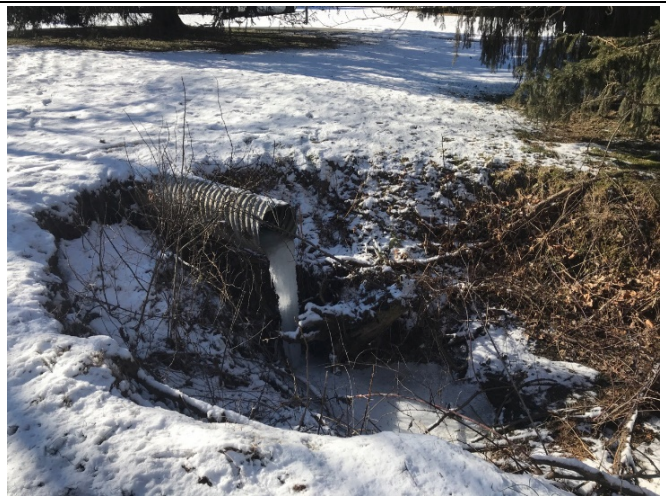
Figure 6: Outfall with highly eroded outfall channel.
