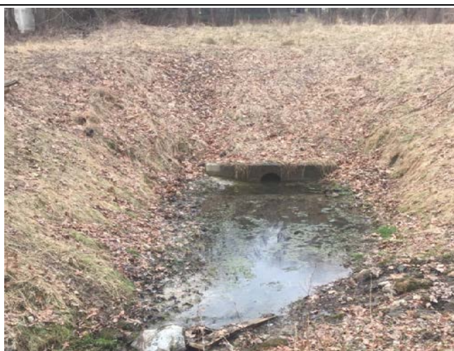
Figure 3: Water in outfall channel is backing up into outfall pipe.
