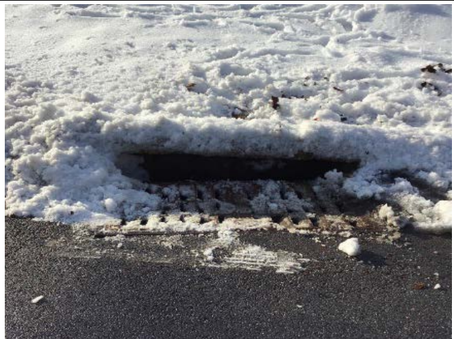
Figure 2: Uneven asphalt in front of inlet at intersection of Michaels Way and Ramblewood Rd.
