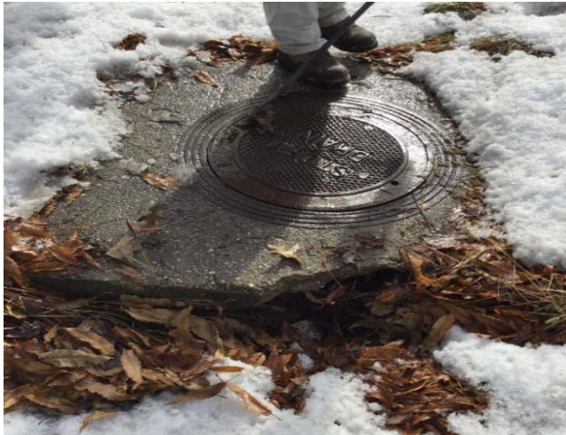
Figure 1: Damaged concrete at inlet.
