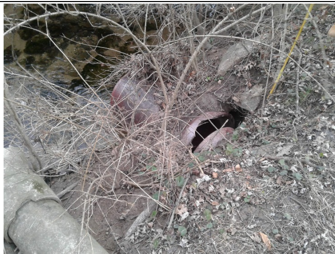
Figure 4: Outfall is broken at joint.
