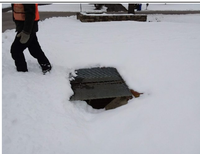
Figure 3: Typical inlet along MacAlpine Road requiring repair.
