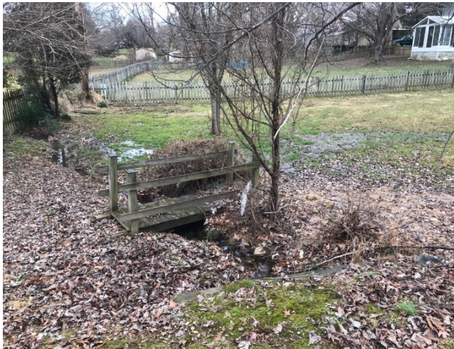
Figure 1: Channel running through back yard at 3134 Hearthstone Rd.
