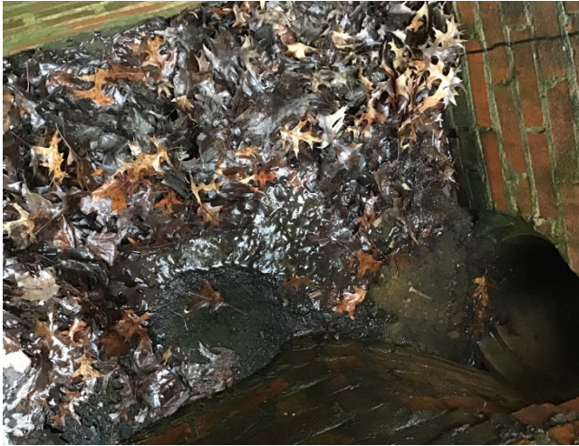
Figure 1: Inlet filled with sediment and debris.
