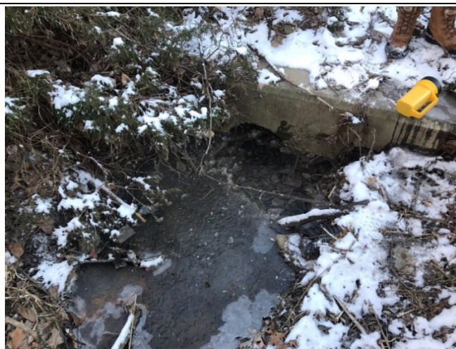
Figure 2: Outfall partially submerged due to sediment and debris buildup.
