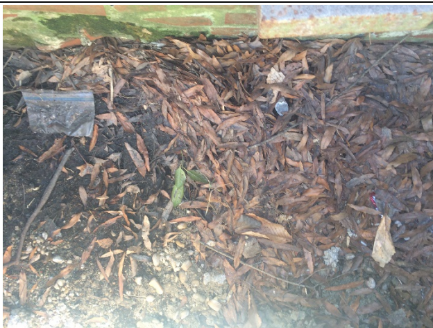
Figure 3: Typical inlet with observed debris.
