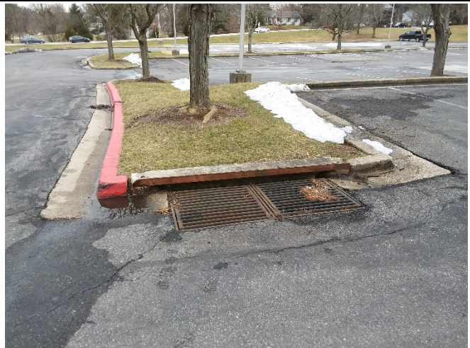
Figure 4: Typical inlet within The Church of Jesus Christ of Latter-Day Saints parking lot.
