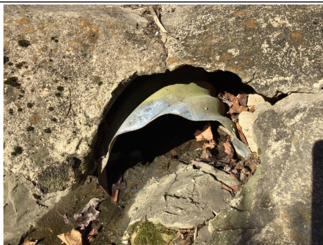
Figure 6: Outfall is deformed and partially buried.
