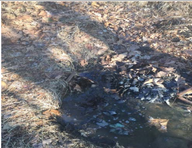
Figure 1: Storm drain outfall is damaged and partially buried.
