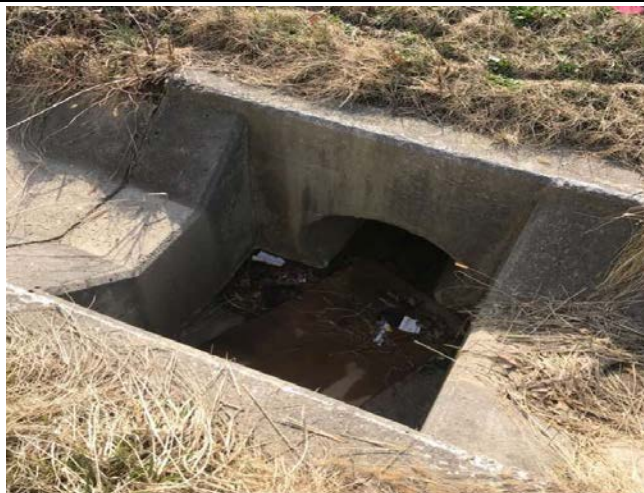
Figure 1: Grate missing from inlet.
