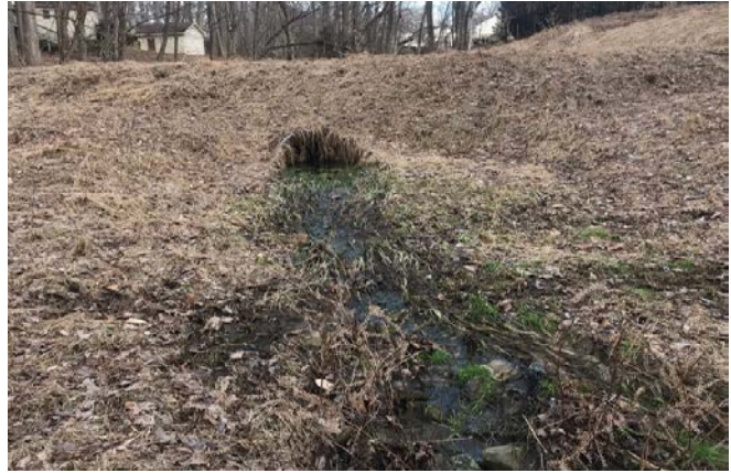
Figure 2: Outfall is partially blocked.
