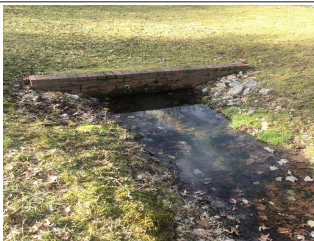
Figure 5: Outfall and downstream channel submerged in standing water.
