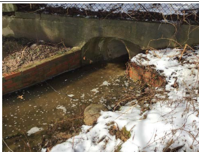
Figure 2: Outfall at upstream end of channel with standing water observed.
