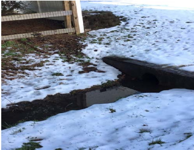
Figure 1: Storm drain outfall channel with standing water.
