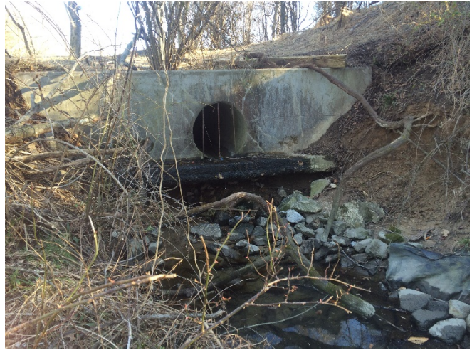
Figure 2: Outfall requiring repair on the campus of Dunloggin Middle School.
