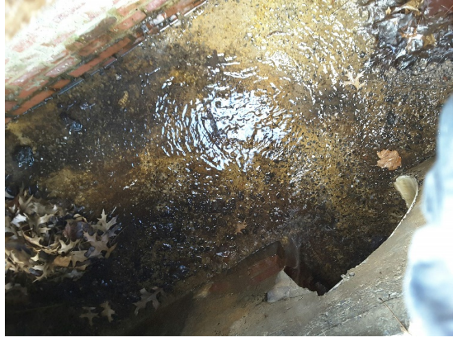
Figure 2: Typical inlet along Westwood Drive with observed debris.
