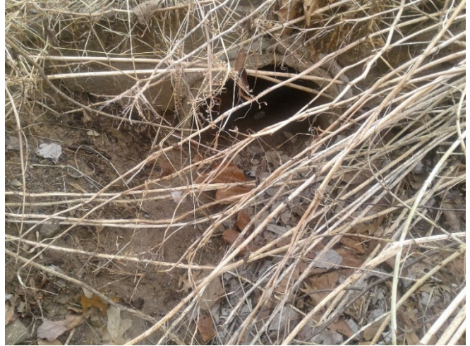
Figure 2: Storm drain partially filled with sediment.
