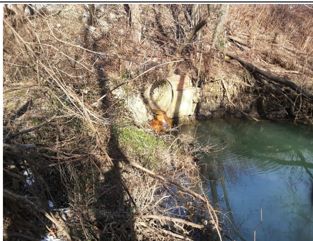
Figure 1: Outfall requiring repair.
