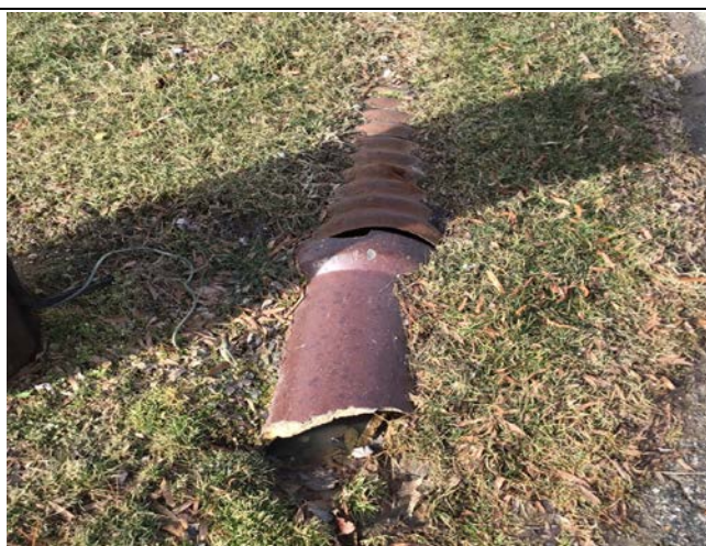
Figure 3: Pipe is disjointed and upstream end could not be located.
