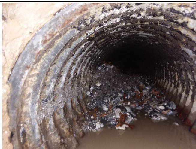
Figure 4: Gravel blocking flow within pipe.
