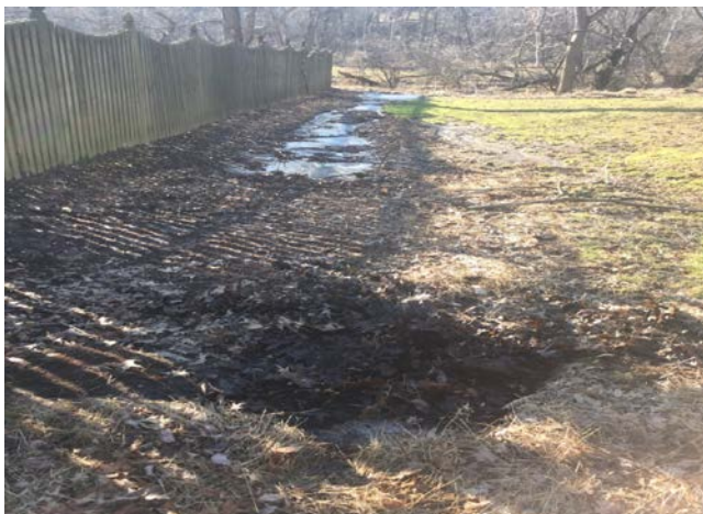
Figure 7: Outfall and outfall channel is buried in sediment and debris.
