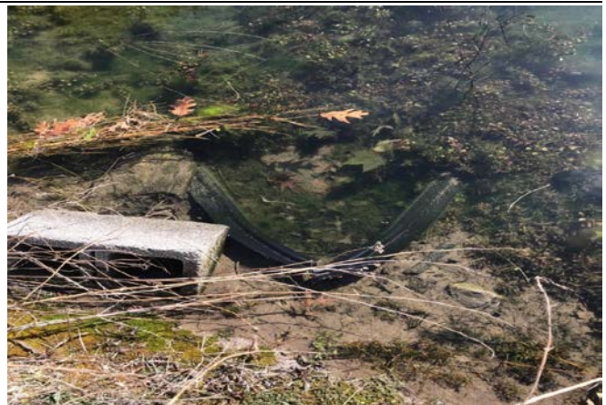
Figure 1: Inflow to facility is submerged and filled with sediment.
