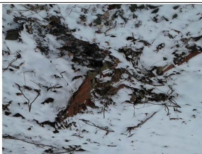
Figure 4: Outfall is collapsed.
