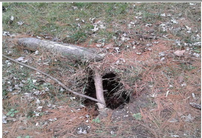
Figure 2: Sinkhole above assumed location of pipe behind houses on Greenway Dr.
