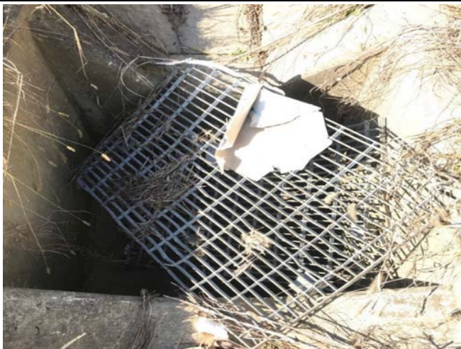
Figure 2: Grate detached from inlet.
