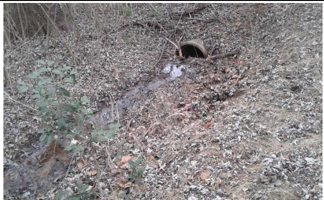
Figure 4: Channel leading up to pipe is filled with sediment and debris.
