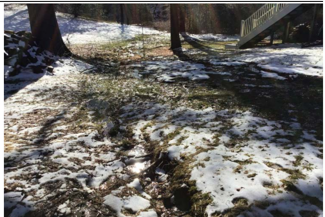
Figure 3: Eroded storm drain outfall channel through homeowner's yard.
