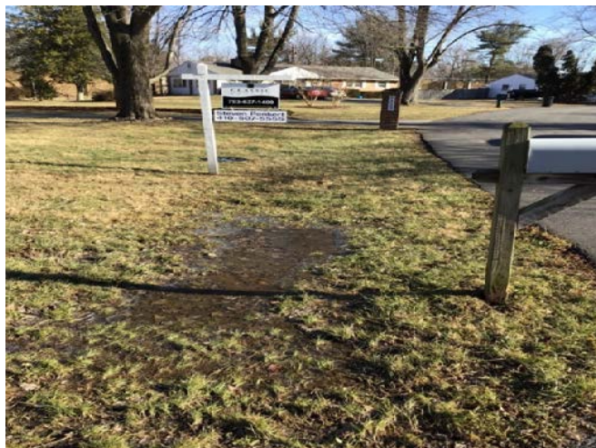
Figure 1: Standing water in roadside ditch along Millbrook Rd.
