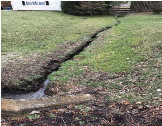
Figure 3: Eroded Outfall Channel.
