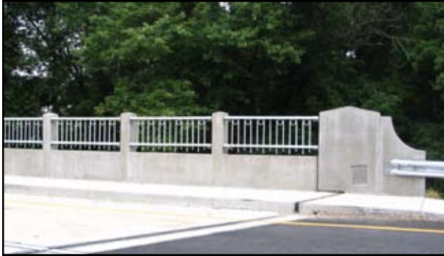
Renovations of the northbound US 1 bridge over the Patuxent River in North Laurel preserves the 1949 historic character of the roadway.
